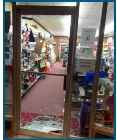
The preferred route of entry for almost half of pharmacy burglaries is through the front door.
